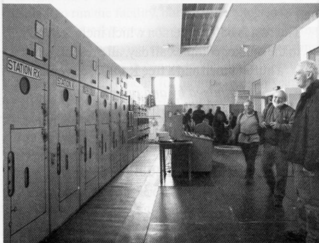
Lovely old generator control panel
